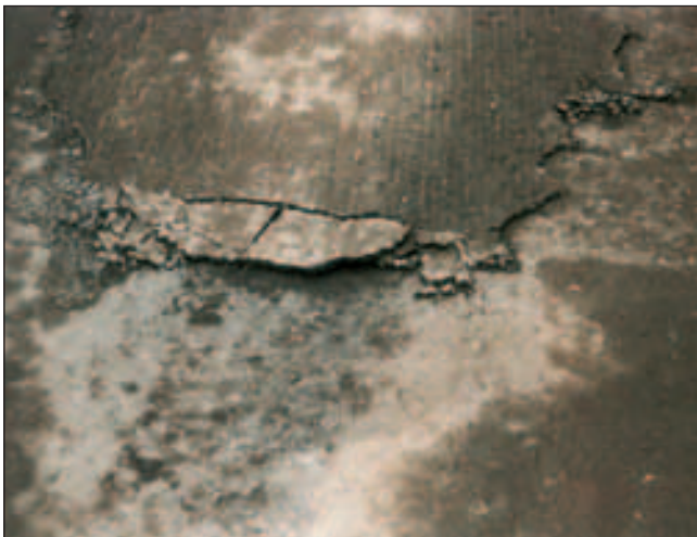
Condition of roads after milling of surface 1996.
